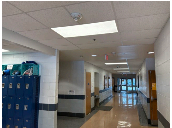
40 - FIRE ALARM SYSTEM DEVICES
