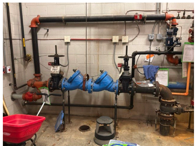
36 - FIRE BACKFLOW PREVENTER
