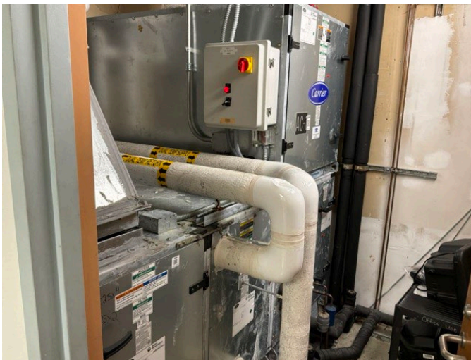
33 - INTERIOR AIR HANDLER
