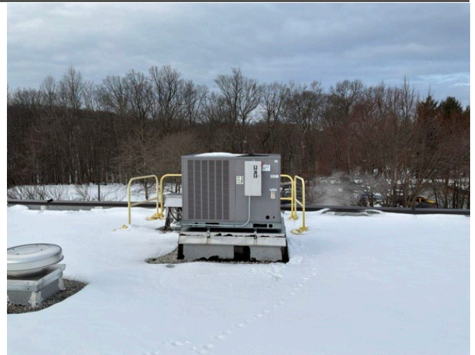
32 - SPLIT SYSTEM CONDENSING UNIT
