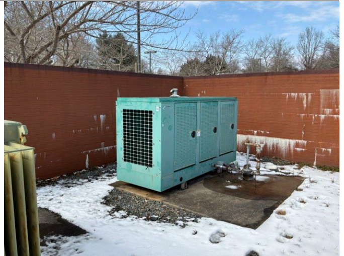
38 - EMERGENCY POWER GENERATOR
