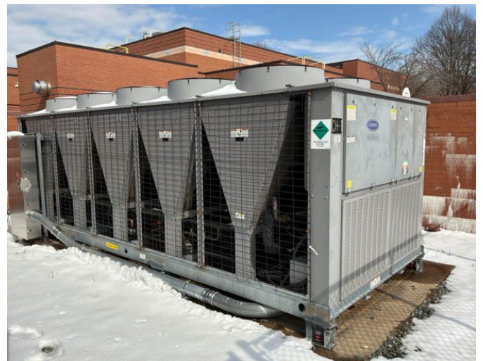
28 - AIR COOLED CHILLER
